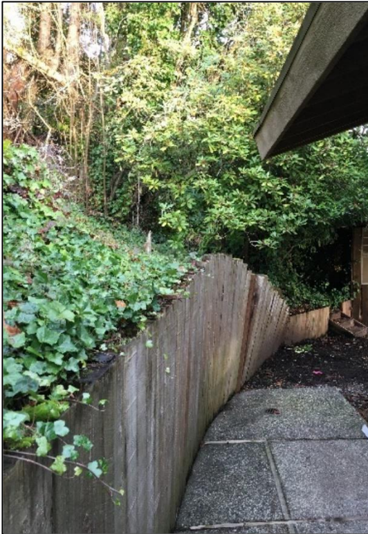
Photograph 1. Looking northeast at the existing yielding wall northwest of the existing residence.
